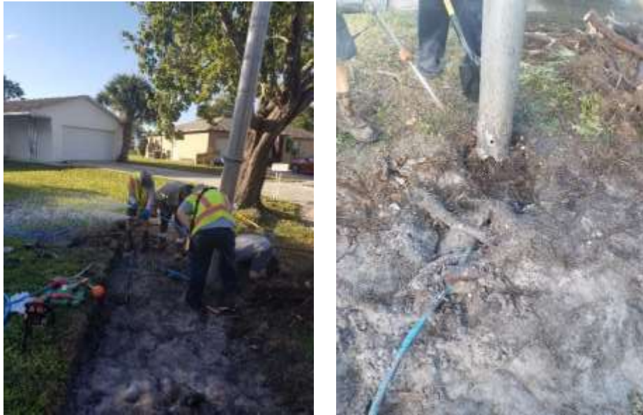
Photo of water service repair damaged by tree roots on Kane Dr.
