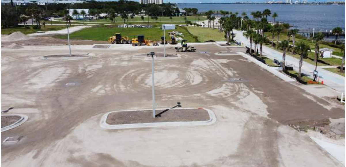
Aerial photos of construction work at Fysh Bar & Grill at Riverwalk Park
