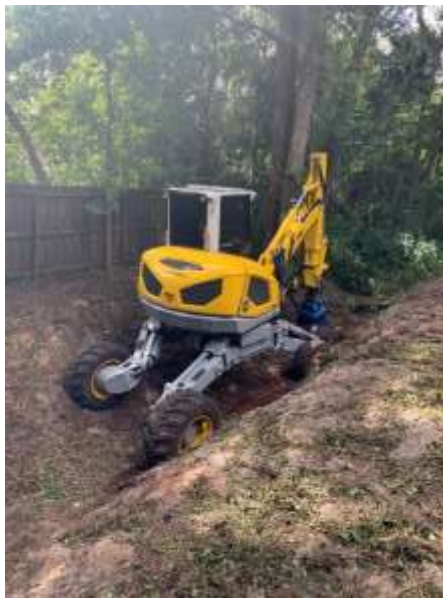
Photo of the Menzi cleaning the ditch along Silver Sands Middle School
