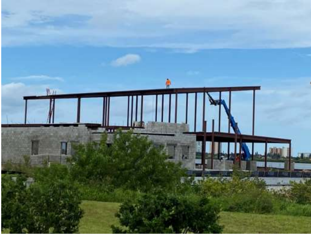
Photo of roof panel construction activity at Riverwalk Fysh Bar & Grill restaurant site
