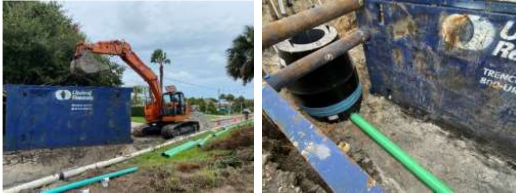
Photo on work being installed on a 8” gravity sewer main for Ponce De Leon Circle in Ponce Inlet
