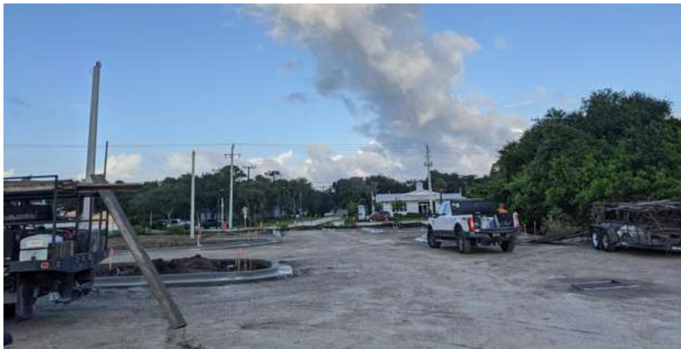
Photo of parking lot construction activity at Fysh Restaurant at Riverwalk Park
