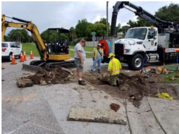
Photo of Field Operations crew repairing the watermain on Willow Run Blvd.
