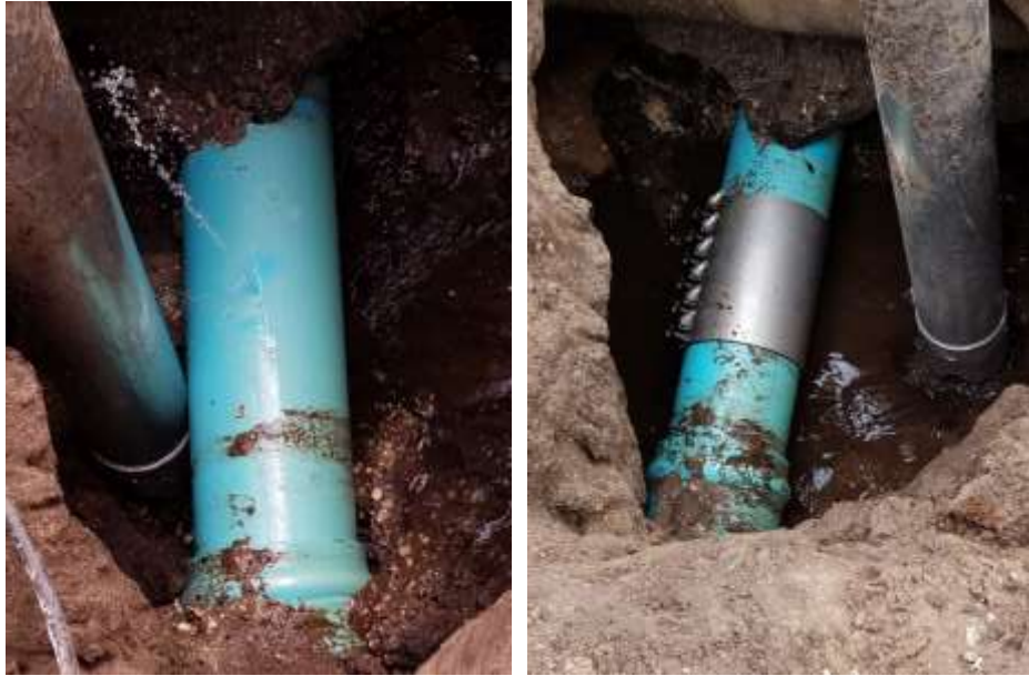
Photo of split “class” pipe on Willow Run that was repaired by Field Operations
