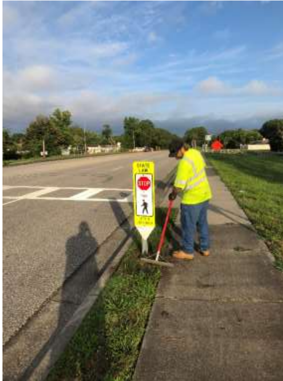
Photo of staff installing a pedestrian signs at the crosswalk on Willow Run at Tracy Dr.
