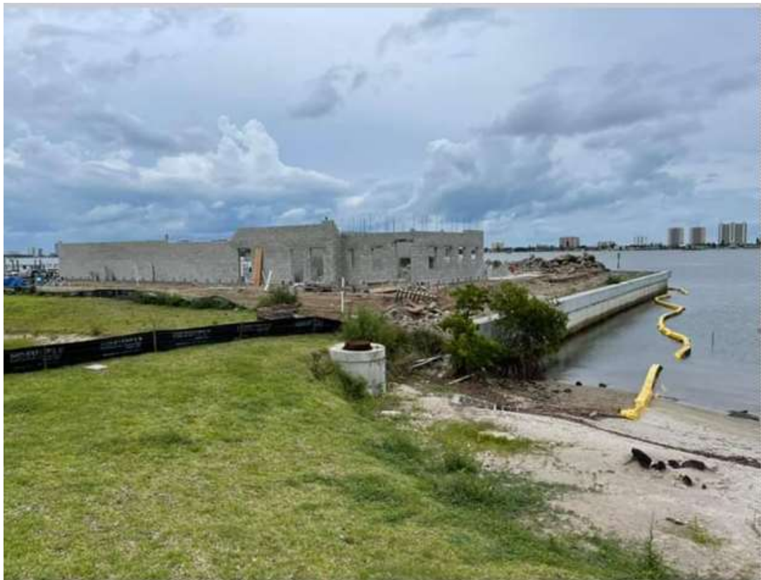
Photo of the concrete masonry unit (CMU) block walls going up for Fysh Bar & Grill Restaurant
