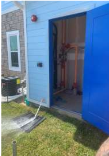
Picture of an inspector test flowing to sound the alarm
