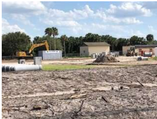
Photo of construction work in progress on Fysh Restaurant at Riverwalk Park.
