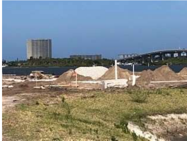
Photo of construction work in progress on Fysh Restaurant at Riverwalk Park.
