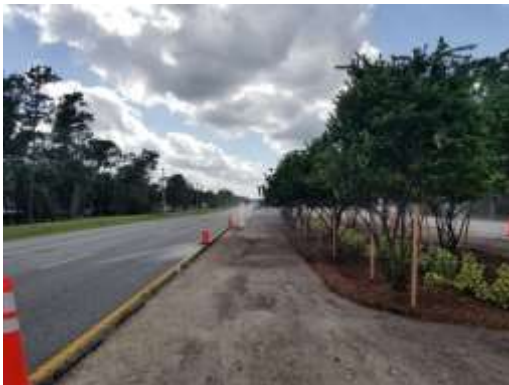
Photo of testing irrigation in median
