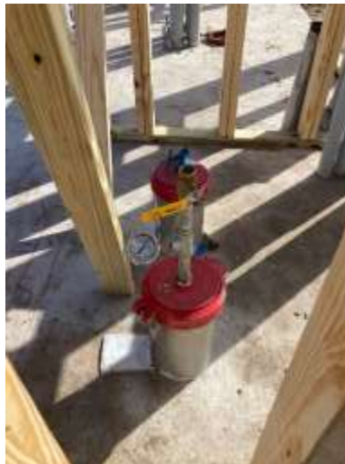
Pic of pressure gauge holding 200PSI on underground FDC pipe
