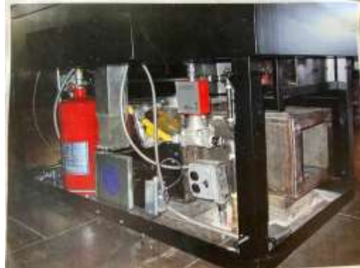
Photo of an example of what table looks like underneath with fire suppression system in place
