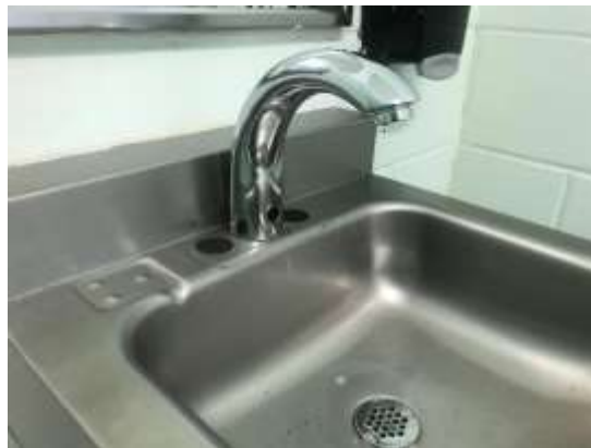
Photo of New Touchless Faucet installed in the Restroom at Causeway Park
