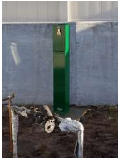
Photo of the new water sampling station installed on Ocean Ave.
