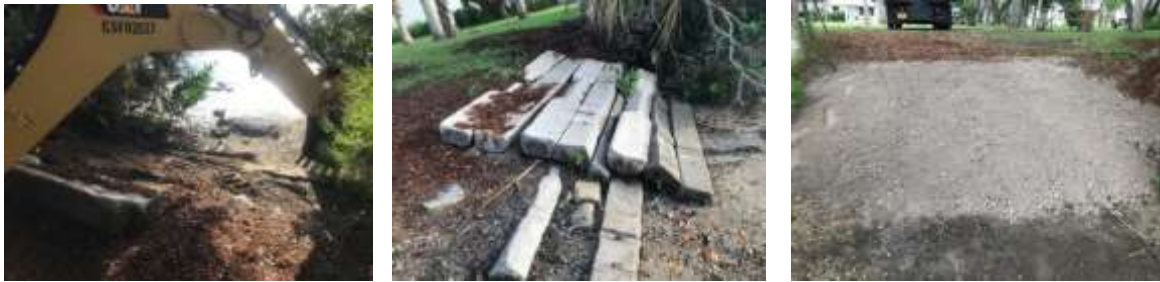
Photos of the before and after the removal of the concrete planks
