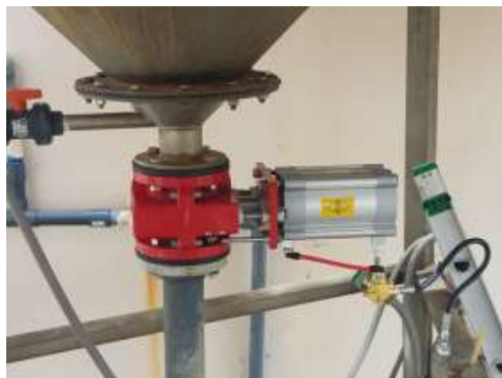
Photo of new pinch valve installed at the WRF
