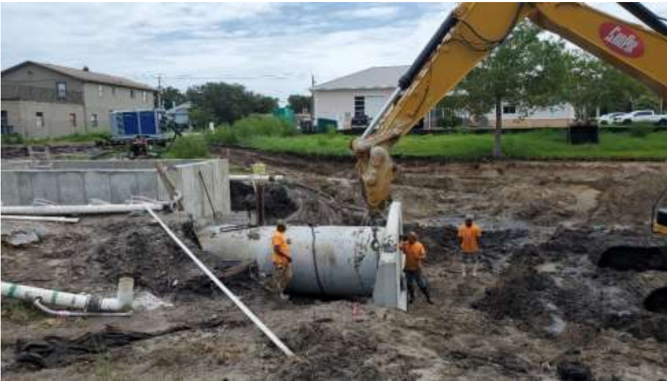
Contractor installing 48"x72" ERCP storm pipe and head wall at the Monroe St. pond
