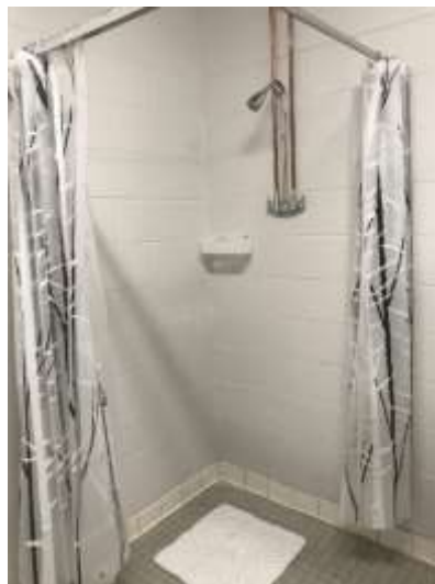
Photo of New Shower that was installed at the DLH City Center Annex
