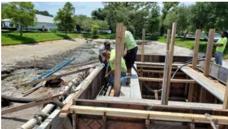
Photos of stormwater pipe installation and new stormwater pump station on the Virginia Monroe project
