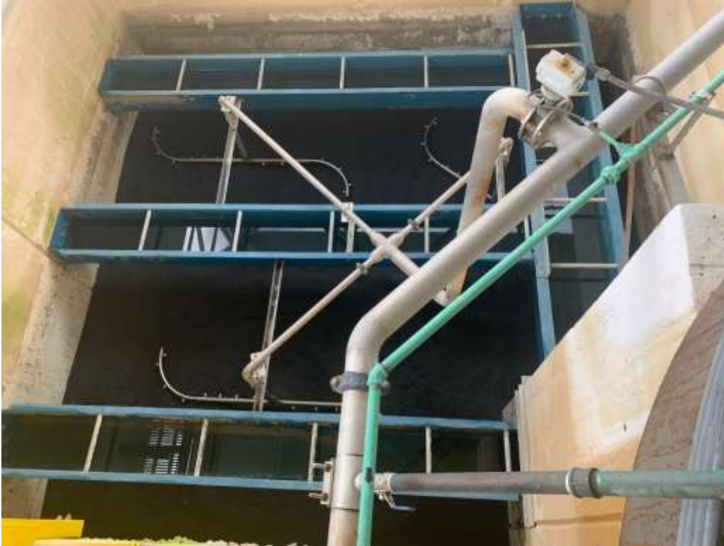
Photo of new filter media installed at the Water Treatment Facility
