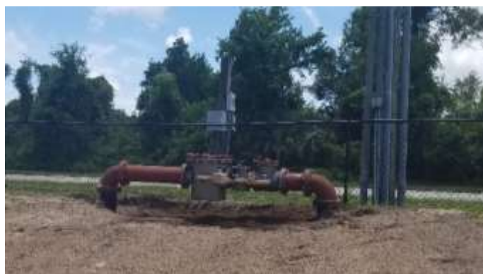
Photos of new 8” backflow installation at Spruce Creek High School this past weekend
