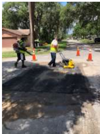
Photo of Staff Paving the corner of Legume Drive and Hamlet Drive
