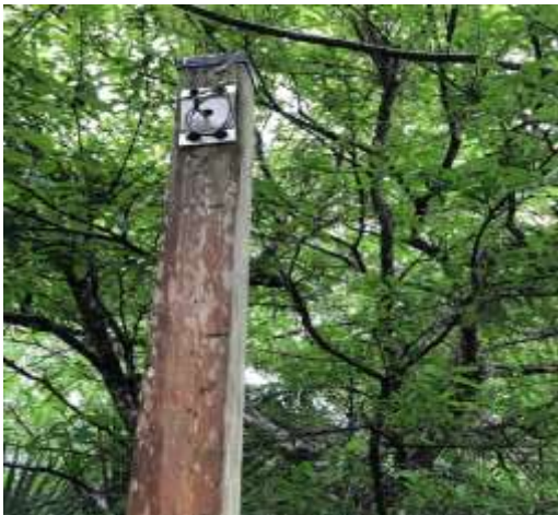
Photo of broken light pole
