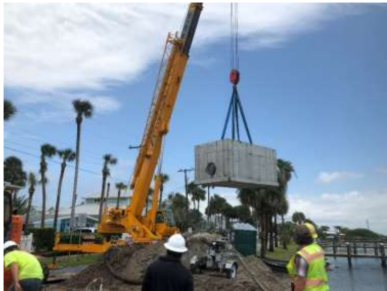
Photo of outfall structure being install on Halifax Dr. at Meeker Street
