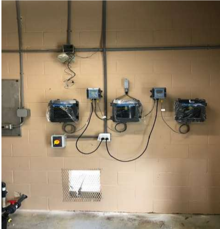
Photo of new chlorine analyzers installed at the WRF
