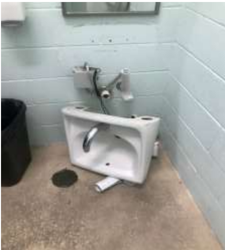
Photo of broken sink
