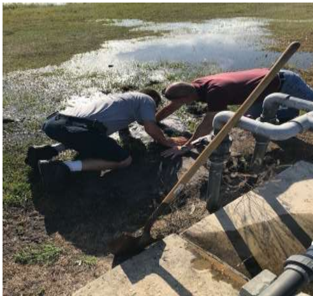
Photo of Chief Plant Mechanic Brent Reed and Raymond Rogers accessing a broken backwash line at the reclaimed lakes.
