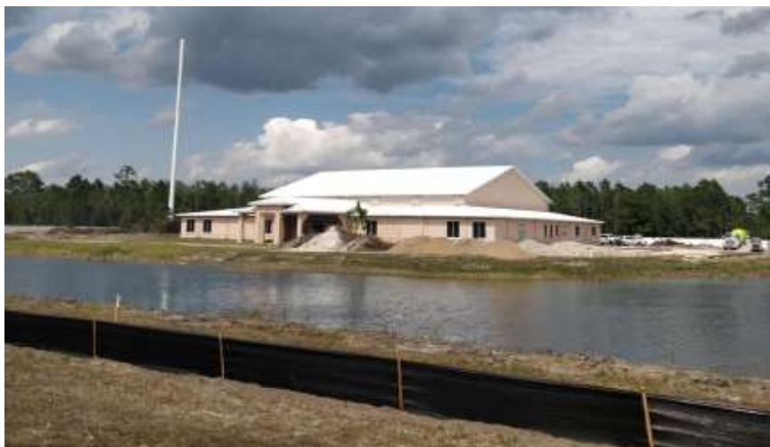
Photo of site work at the property located on the northeast corner of Madeline Avenue and Williamson Blvd.
