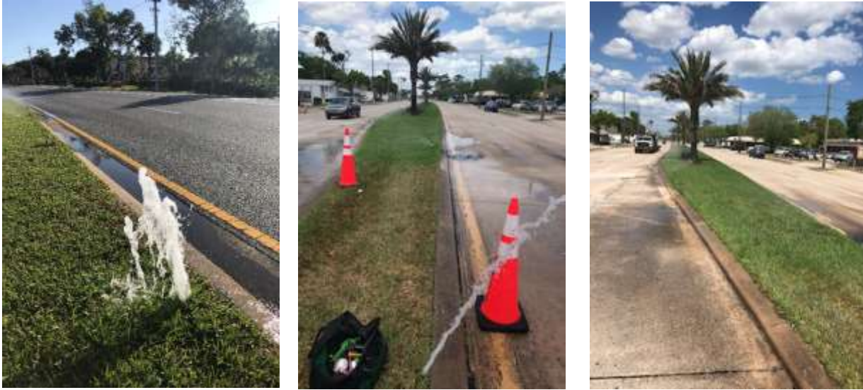
Before and After Photos of an Irrigation Break on Ridgewood Ave.
