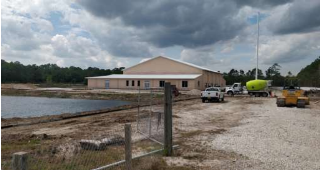
Photo of site work at the property located on the northeast corner of Madeline Avenue and Williamson Blvd.
