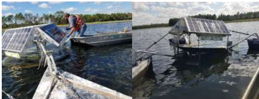
Photo of Technician installing a new battery in a SolarBee at the reclaim lakes
