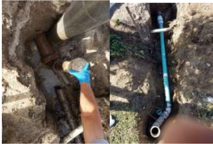
Photo of broken clay sewer line that was repaired with a PVC line
