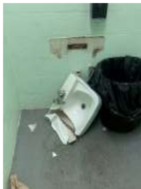
Photo of the broken sink
