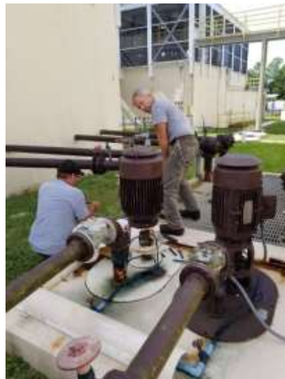
Photo of Randy and Jeff working on a sludge valve at the WTP.
