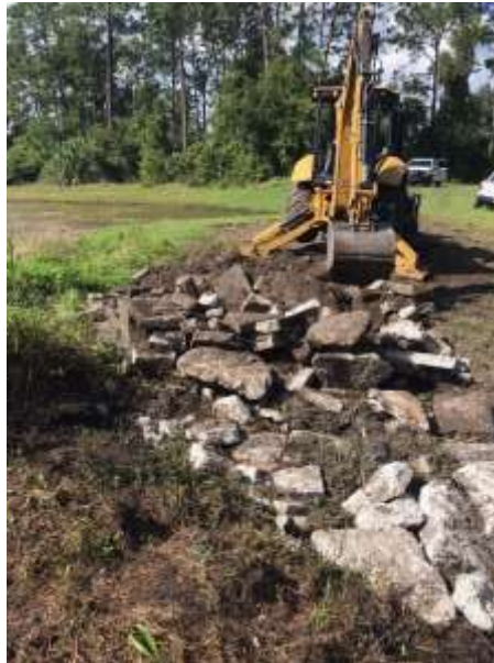
Photo of large washout filled with rubble
