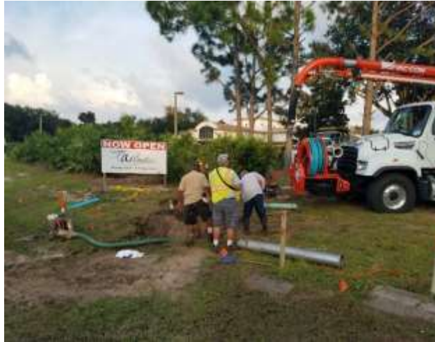
Photo of Field Ops staff repairing a 4-inch valve on Dunlawton Ave
