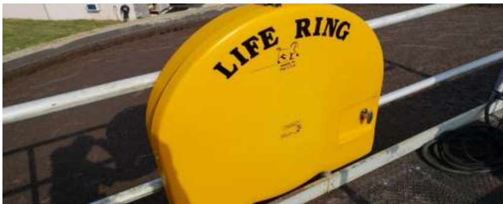
Photo of new life rings installed around the Water Reclamation Facility
