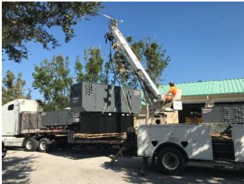
Photo of new generator at Fire Station 74
