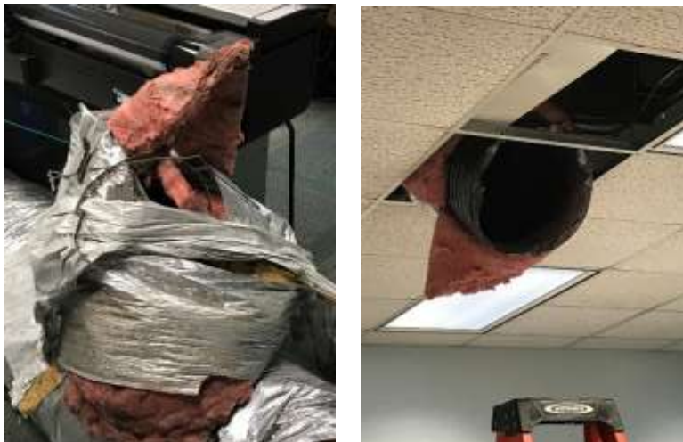
Photos of damaged ducts in Community Development
