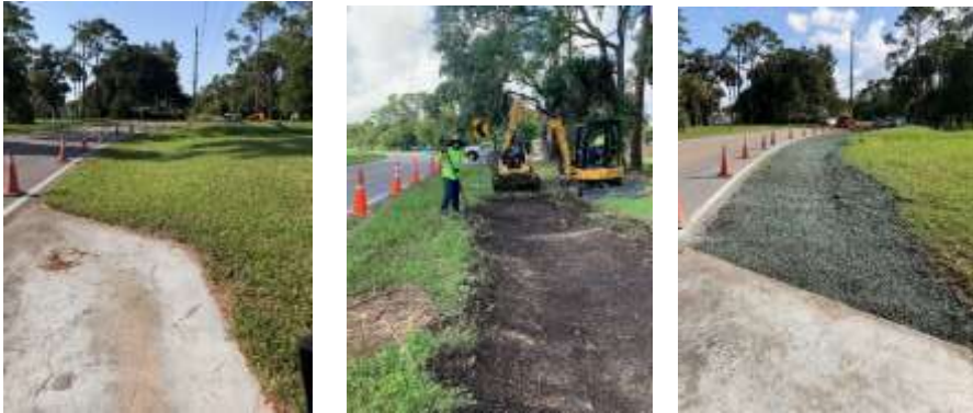
Before, During, and After photos of swale restoration on Spruce Creek Road
