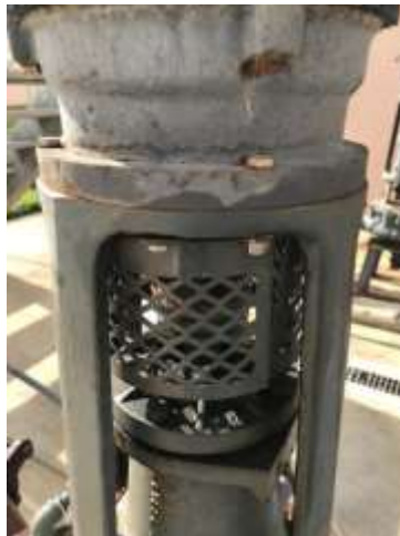
Photo of a new safety guard installed on a sludge pump at the WRF
