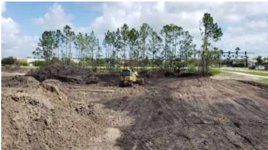
Photo showing clearing and grading of the two outparcels adjacent to the Springs Apartments.
