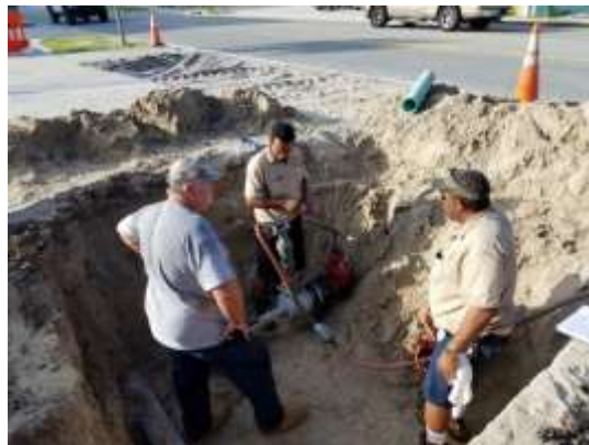
Photo of Robert, Derrick, and Alex performing a water tap on Atlantic Ave.
