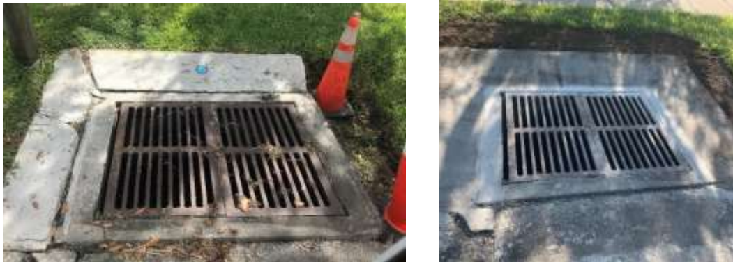
Before and After photos of repair catch basin apron on Wimbledon Ct.
