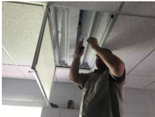
Photo of employee inspecting the facility lights
