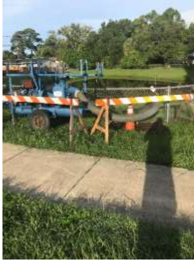
Photo of a portable pump stage on Isabelle Avenue
