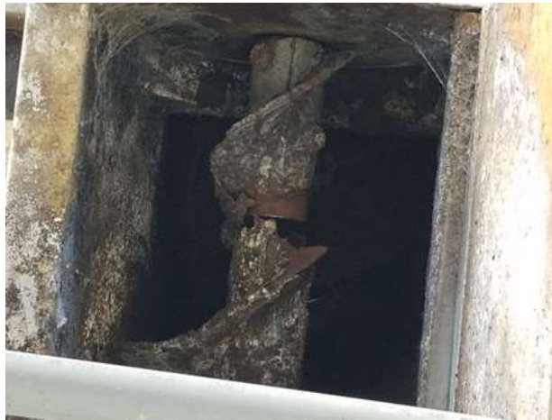
Photo of broken biosolids conveyor at the WRF
