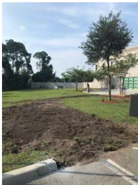
Photo of removed sidewalk at the Police Department
