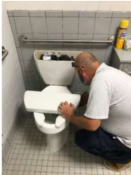
Photo of employee working on the plumbing at the DLH City Center Annex
