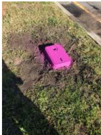
Photo of new irrigation box on Nova Road
